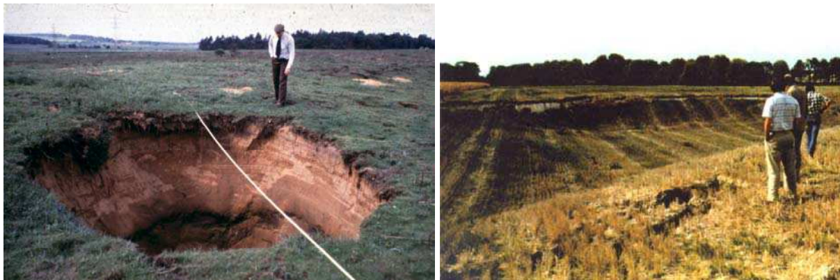
Figure 4. Example of a sinkhole (on the left) and of a general collapse (chalk mine on the right).
