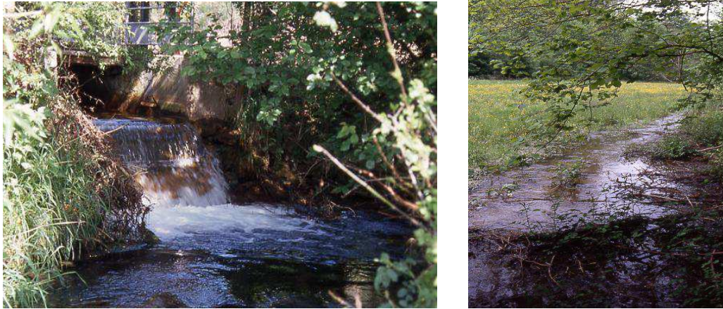
Figure 2. Discharge through an adit (left) and development of a wet zone close to an other adit (right).
