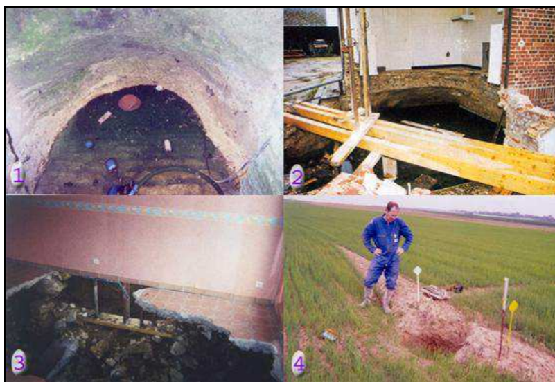
Figure 3: (1) Flooded cellar; (2 & 3) Collapses of buildings due to undermining cavity failure; (4) Backfill run out of an old chalk mine.
