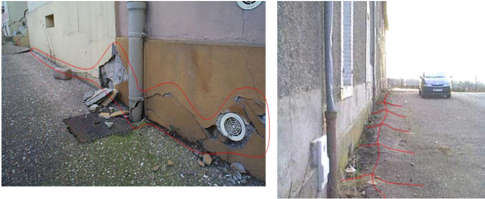
Figure 2: Example of serious structure damages due to subsidence – Iron mine – Lorraine – France
