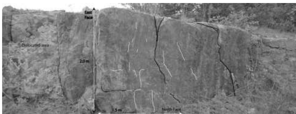
Figure 17: View of the rock mass, it presents a dislocated area on the left, and major discontinuities are in black and superficial are in white.
