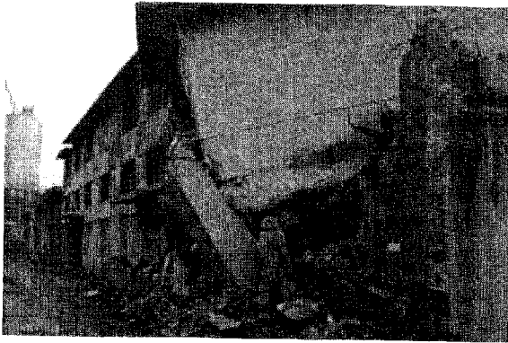
Fig. 2: Building collapse due to insufficient reinforcement.
