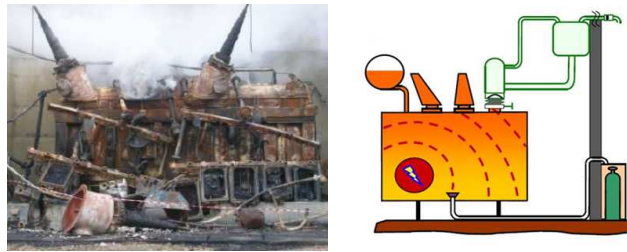
Figure 1: Example of transformer explosion (left) and schema of a transformer and wave propagation in oil bath (right) (source ENEDIS-SERGI).
